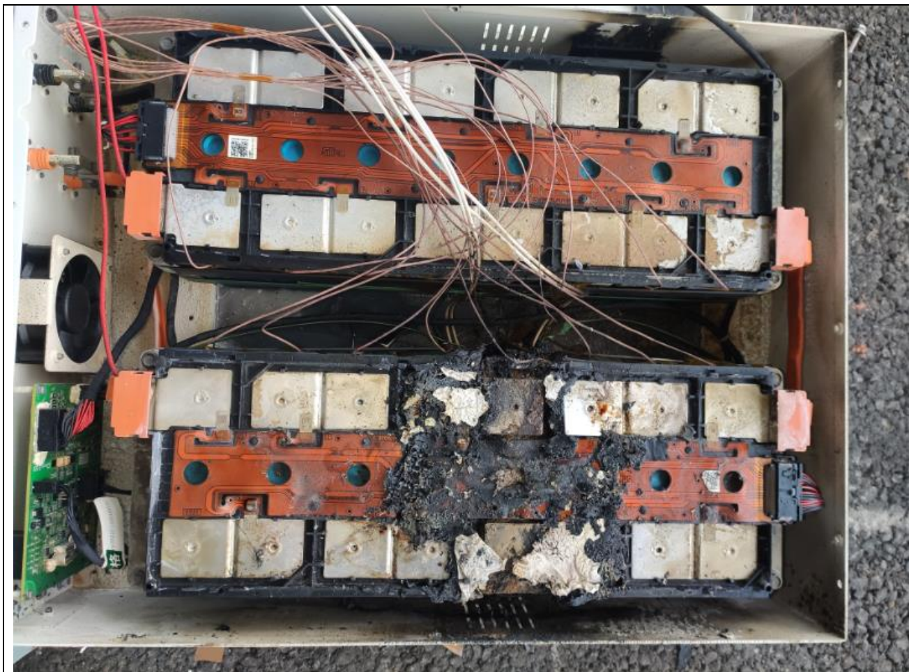
Figure 9a. View of cell that exhibited thermal runaway after test.
