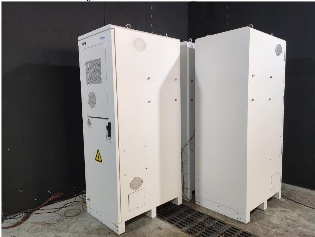
Figure 21a. Photo 02 of after test_ BESS units
